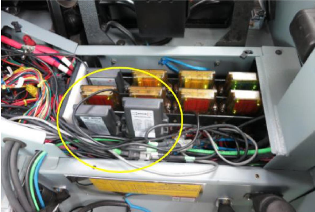
Figure 3.4.2-1. Pierce 1901 VDR installed in cab
